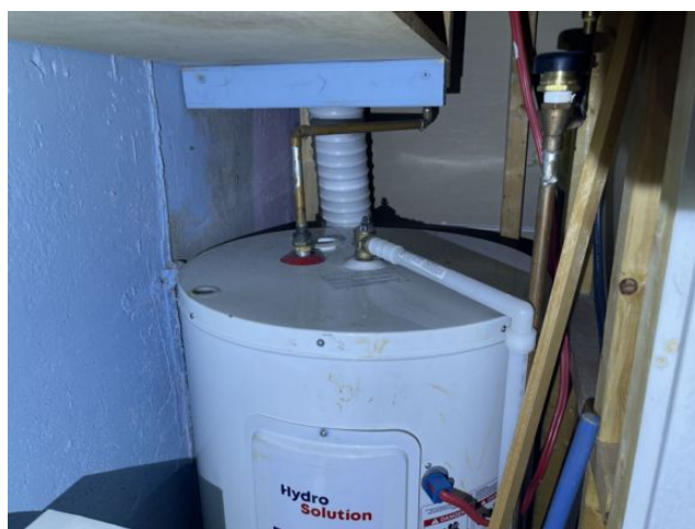
Chauffe-eau en location
